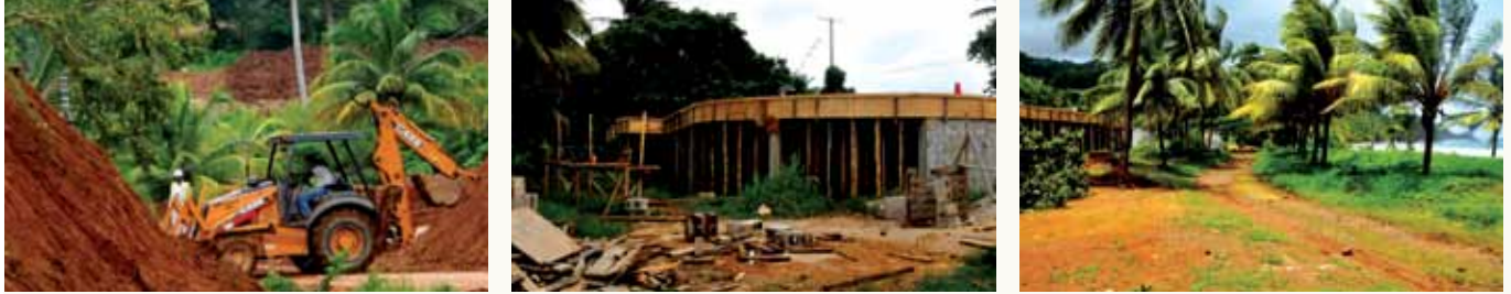
Left: Infrastructural Development, Pond Case to Melville Hall Road Improvement Project. Center and Right: Construction of Inn at Castle Bruce
